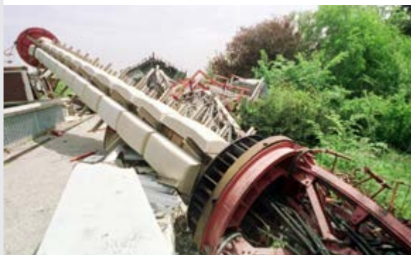
Figure 2.60. The collapsed TV tower on Mount Avala. Photo credit: Rade Prelić.
